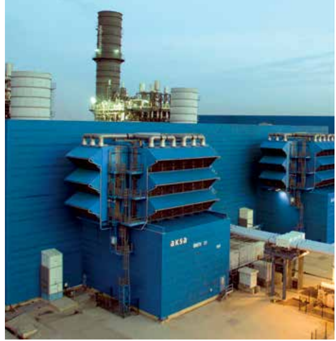
Ali Metin Kazancı Antalya Natural Gas Combined Cycle Power Plant
